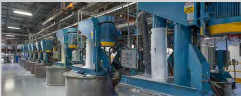
Computer controlled mixing tanks
